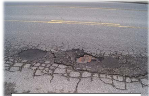
Cracking pavement along Park Avenue
