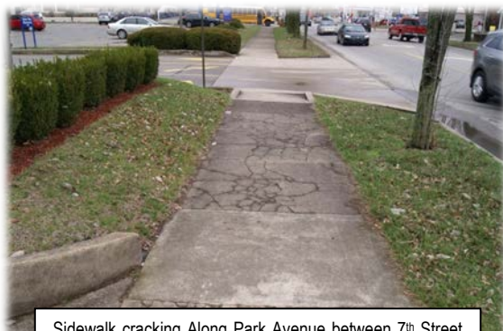
Sidewalk cracking Along Park Avenue between 7 th Street and 8 th Street
