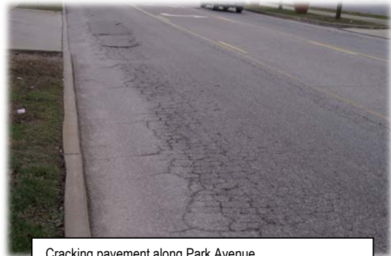
Cracking pavement along Park Avenue
